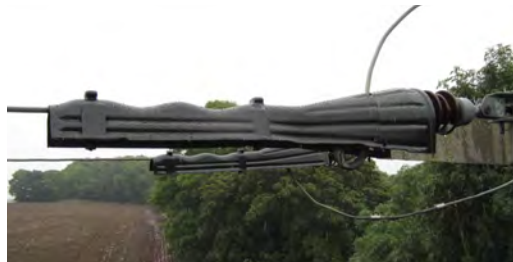
BCIC-TEN-01: Tension Insulator application
