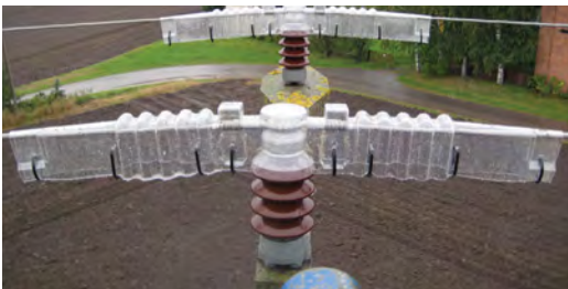
BCIC-1217-TR: Post Insulator application
