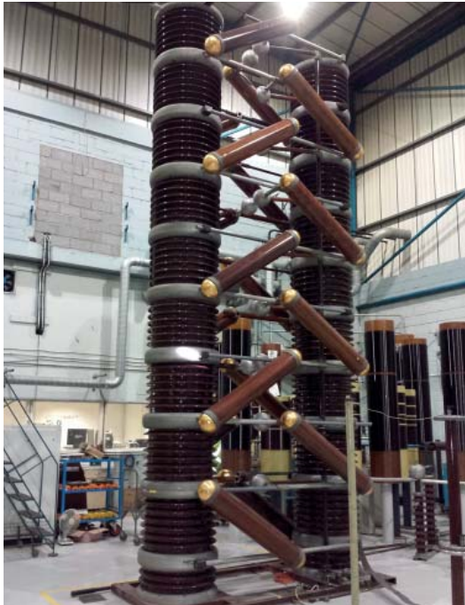
Impulse generator 1.65 MV
