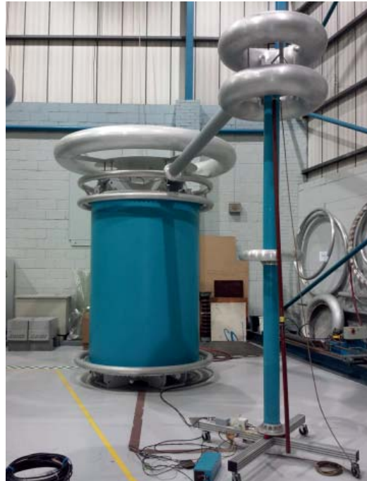
500 kV power transformer with PD testing
