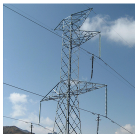
Transmission line arresters
