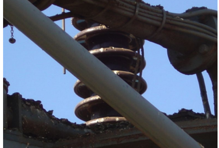
Figure 3. Guano build-up on suspension insulator and on substation equipment.
