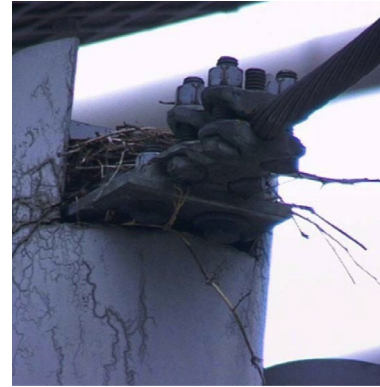
Failure by tracking
