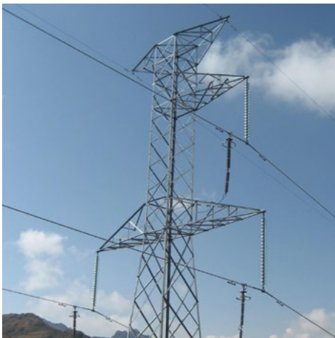
Transmission line arresters
