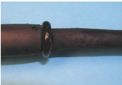
NOT ACCEPTABLE Excess adhesive flow /180
