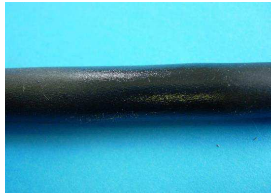
NOT ACCEPTABLE Tubing scorched
