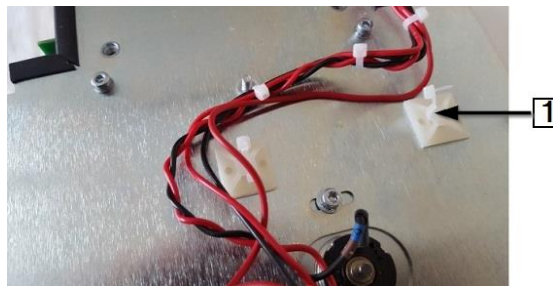
Fig. 57 : Tie-wrap connection on the processor
