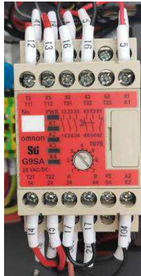
Fig.40 Safety Relay (KS1)
