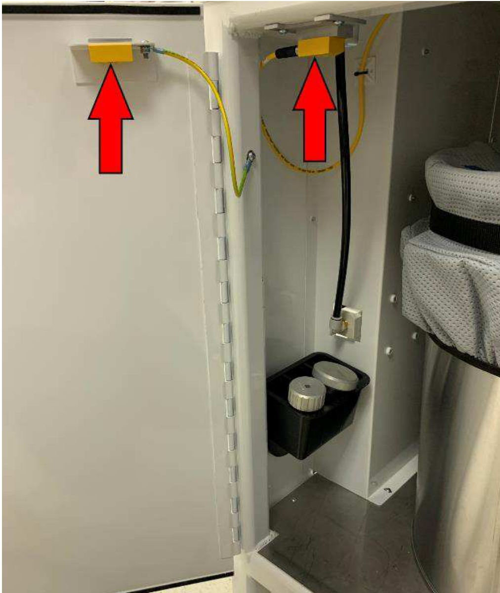
Figure 10: Scrap door safety interlock (open)
