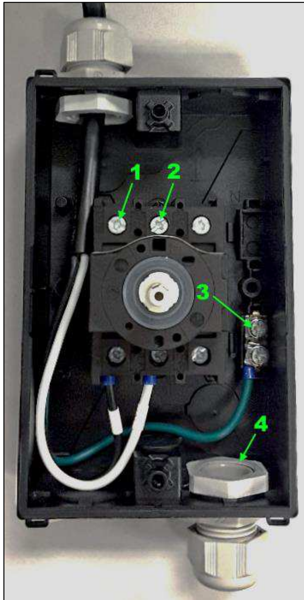
Figure 47: Interior of disconnect enclosure
