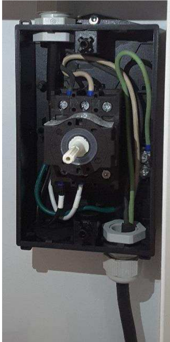
Figure 48: Disconnect enclosure with power cord installed
