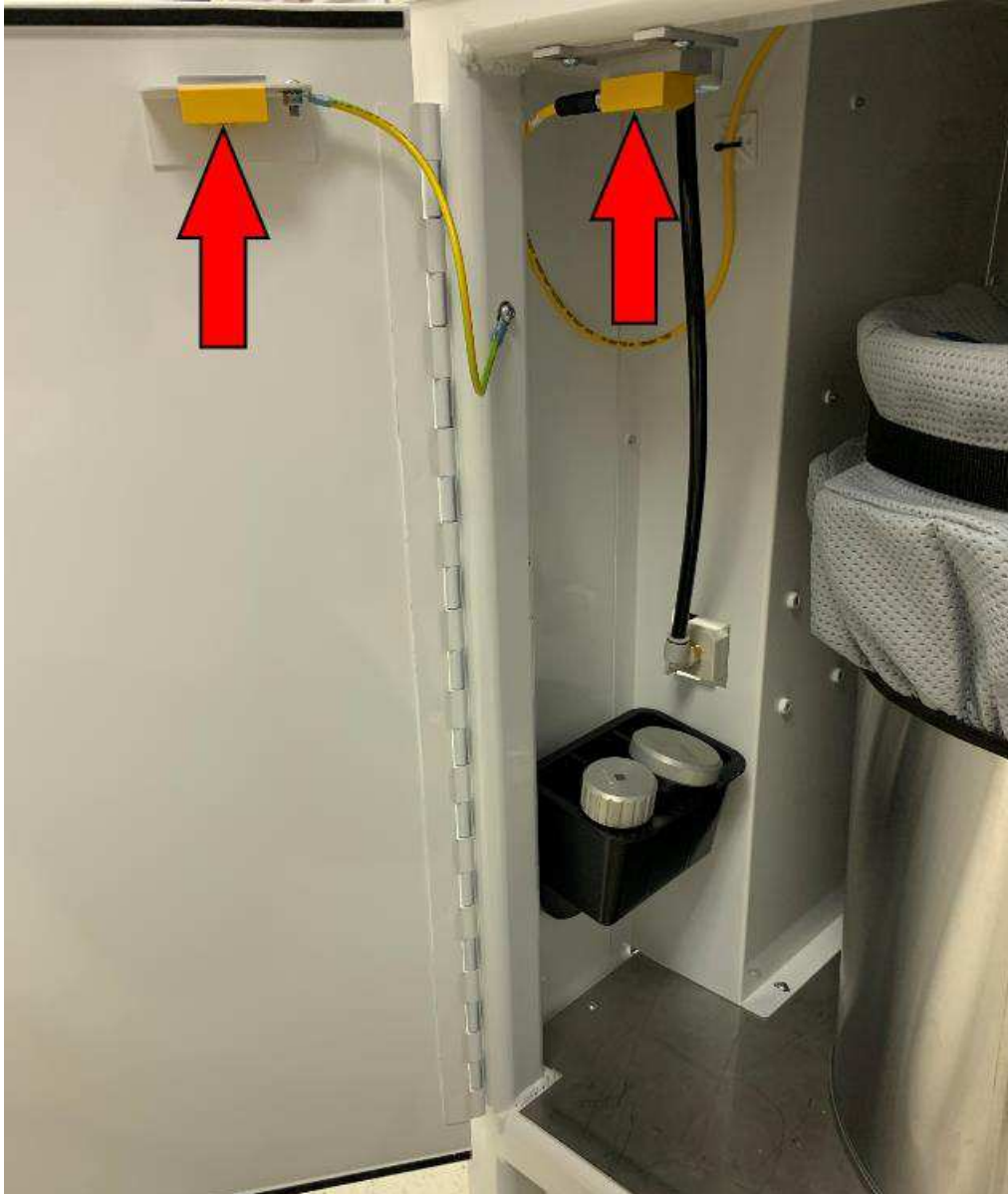
Figure 10: Scrap door safety interlock (open)
