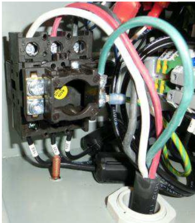
Figure 11: Power disconnect switch
