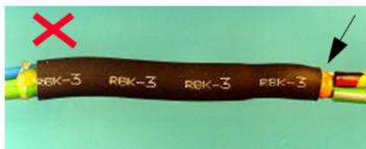
4. Tubing off centre and wire exposed
