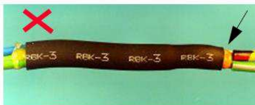
4. Tubing off centre and wire exposed
