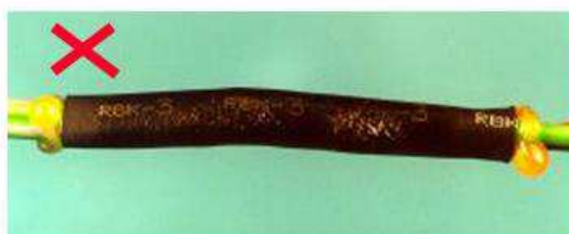
2. Overheat of tubing
