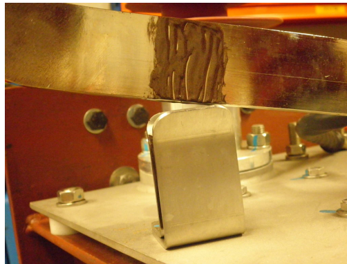
Figure 23: Example of copper slip grease applied to earthing arms on VESA 101 where it enters the earth rest clips.
