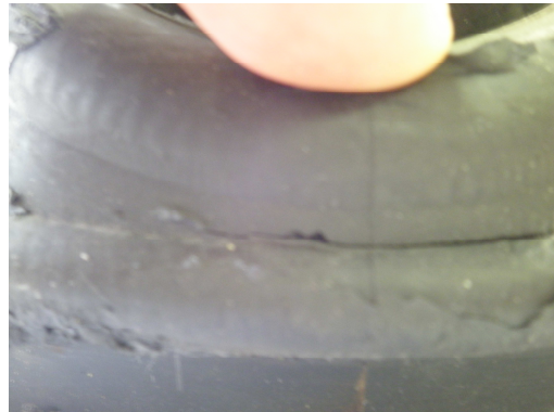
Figure 21: Example rubber gaiter damage
