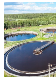
Waste and Water treatment
